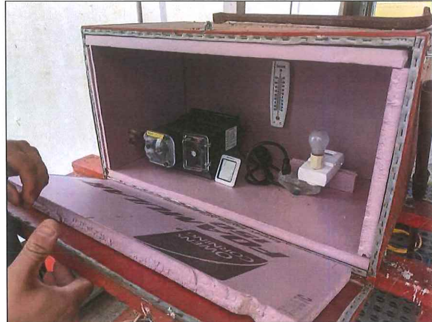
Temporary Chemical Feed System
