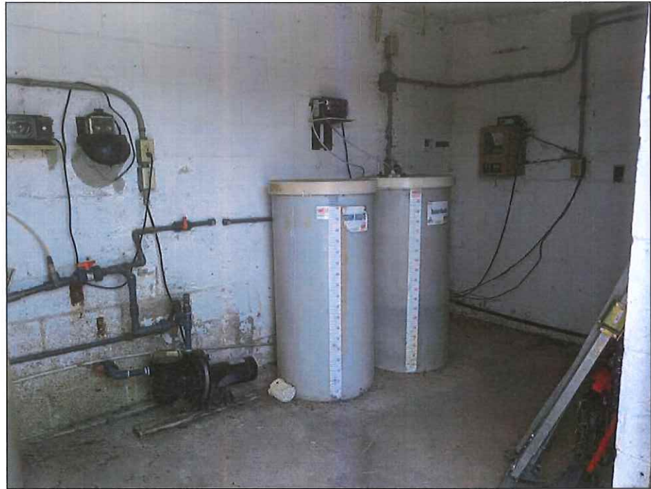
Existing Disinfection System
