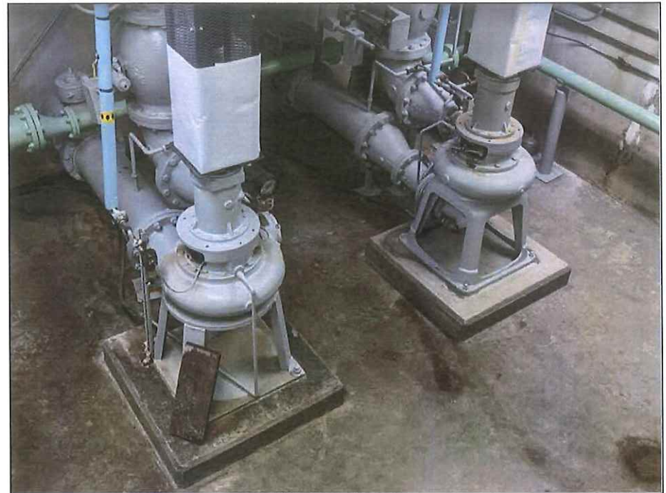
Example of New Raw Influent Pumps
