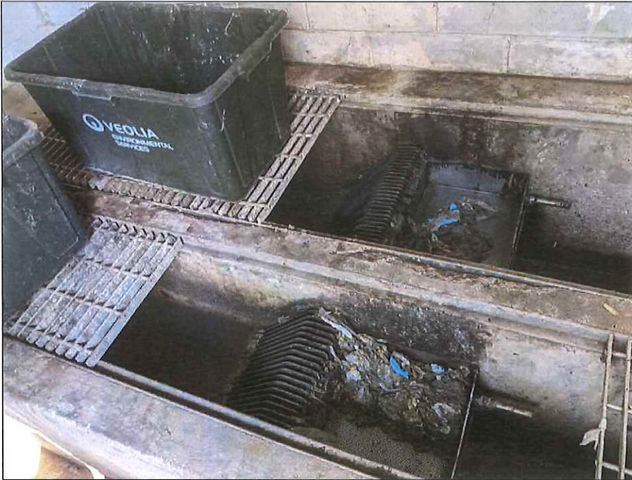
Existing Screen – Manual Cleaning
