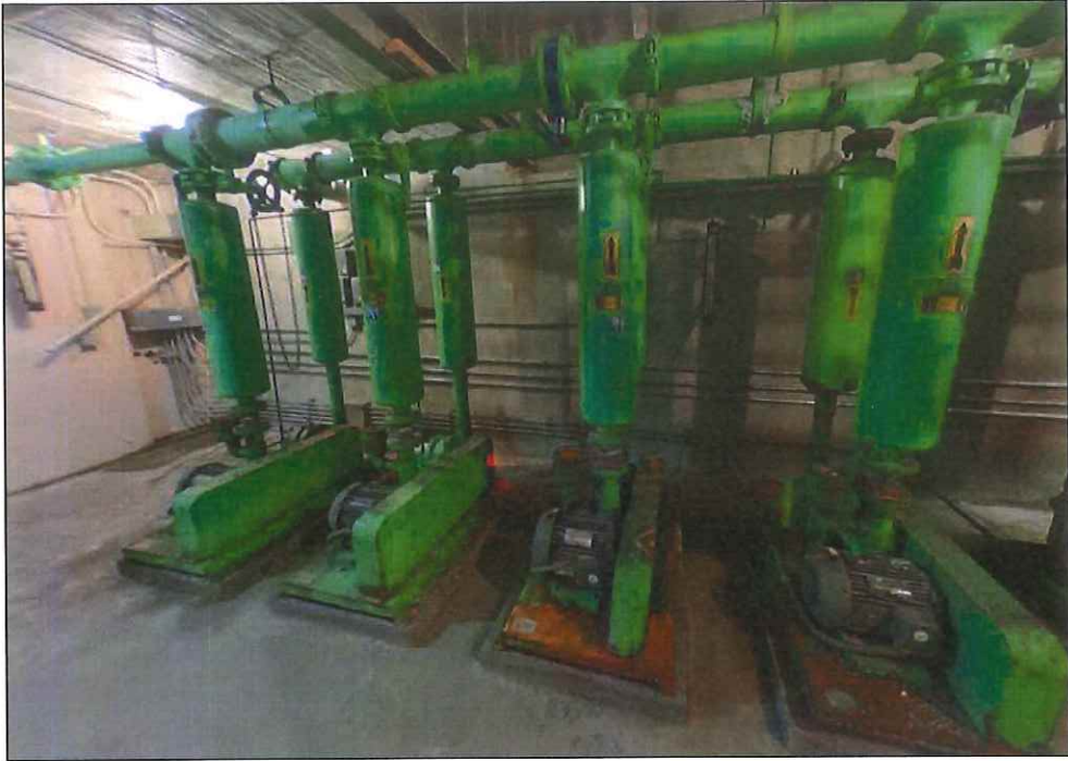
Existing Aeration Blowers
