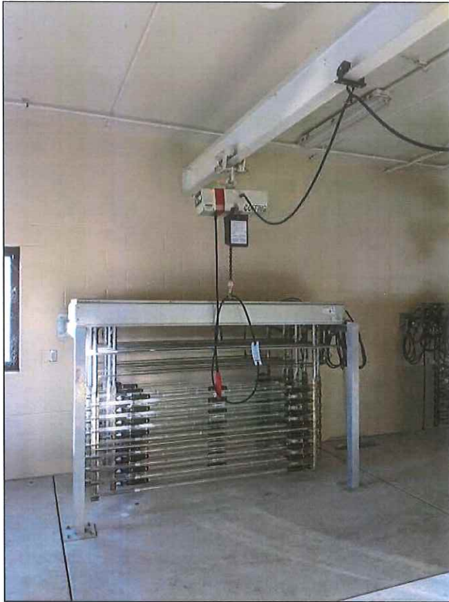
Example of New Disinfection System
