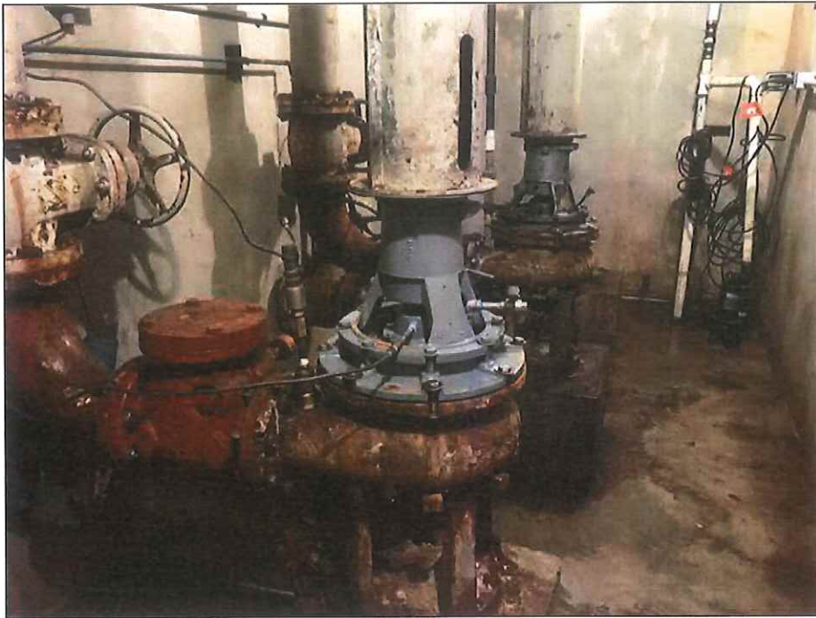
Existing Raw Influent Pumps
