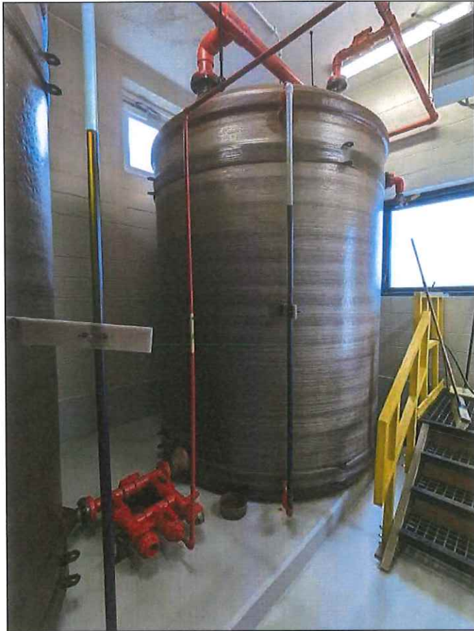
Example of New Chemical Feed System
