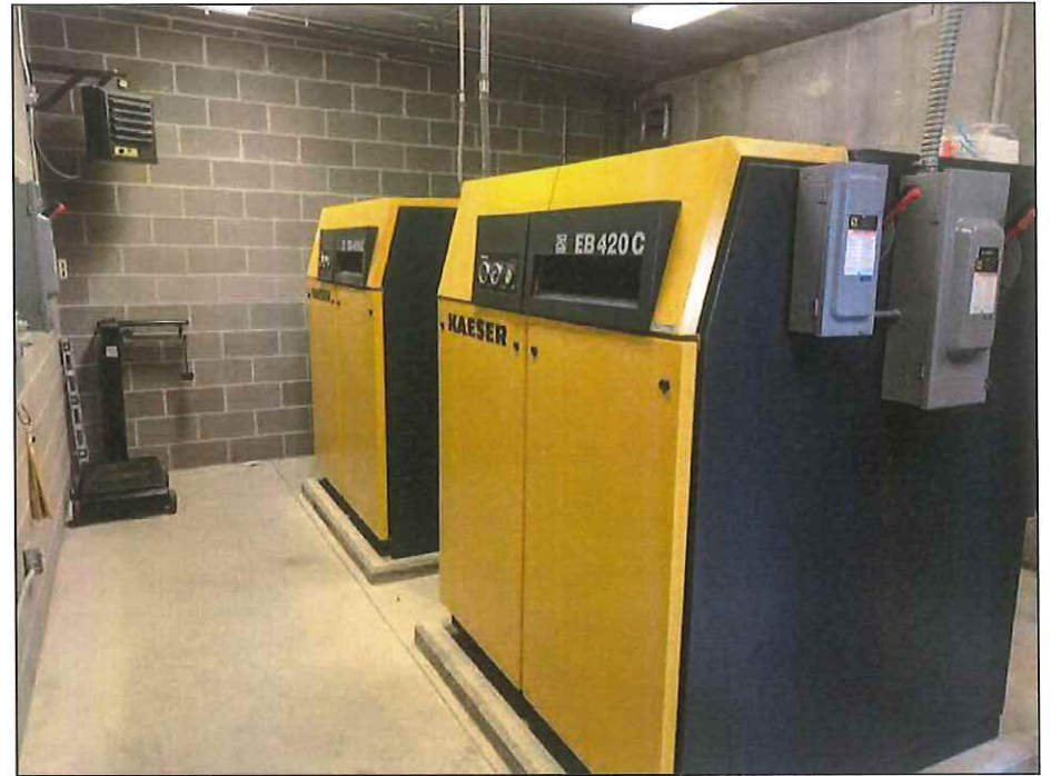
Example of New Aeration Blowers
