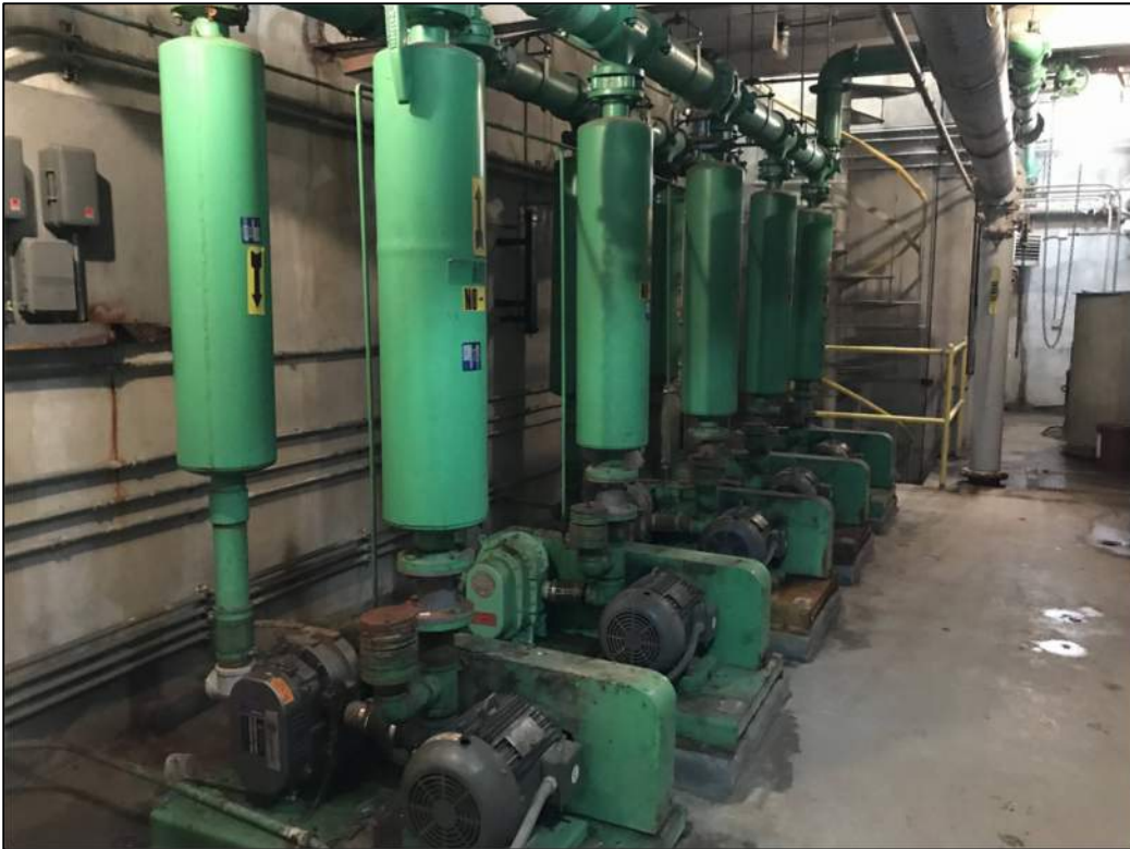
Figure 4. Aeration Tank and Aerobic Digester Blowers
