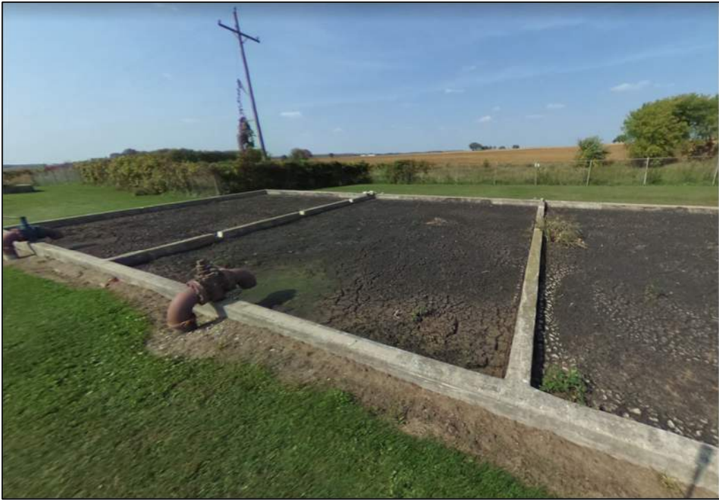
Figure 7. Sludge Drying Beds
