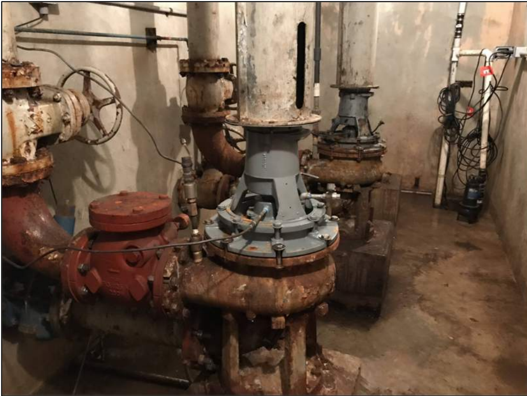
Figure 1. Raw Wastewater Pumps
